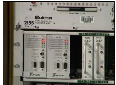
Video image processor, installed in controller cabinet
