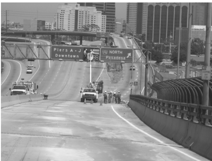
Gerald Desmond Bridge closed to traffic while crews repair concrete deck spalls, stripe, and install overhead speed feedback sign. View from 6% east-bound down grade.
