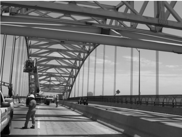
Westbound traffic lanes of Gerald Desmond Bridge are closed while workers repair upper cable restraint plates.
