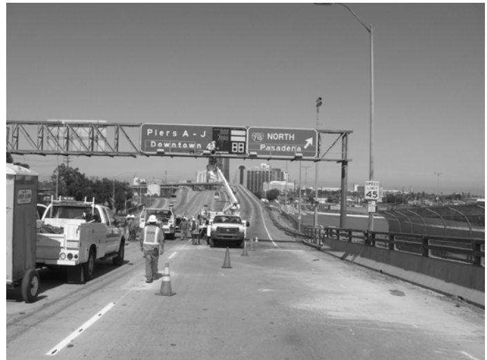
Gerald Desmond Bridge closed to traffic while crews install overhead speed feedback sign.
