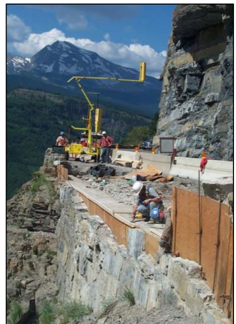
Removal of existing stone masonry guardwalls on the Going to the Sun Road occurred last summer.
